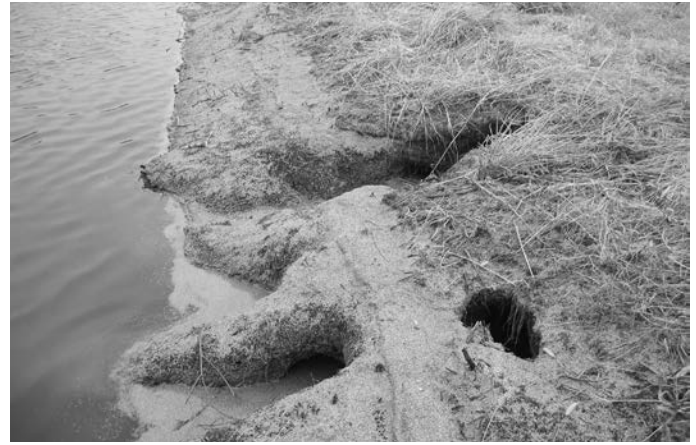
Figure 2. This neglected lagoon shows animal damage and poor grass care.
